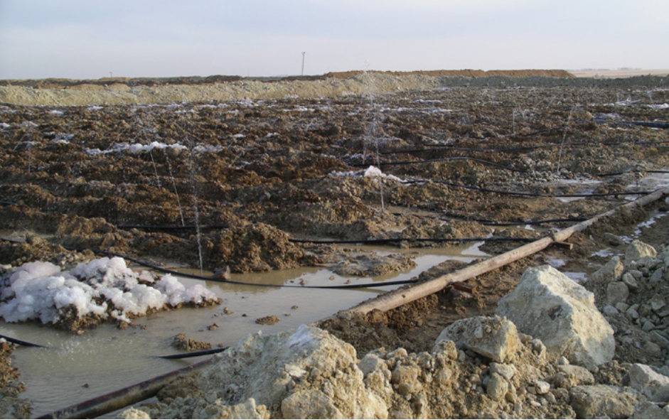
Sprinkling system on the top of the ore heap. The heaps are sprinkled with lixiviant through a top distribution system.
