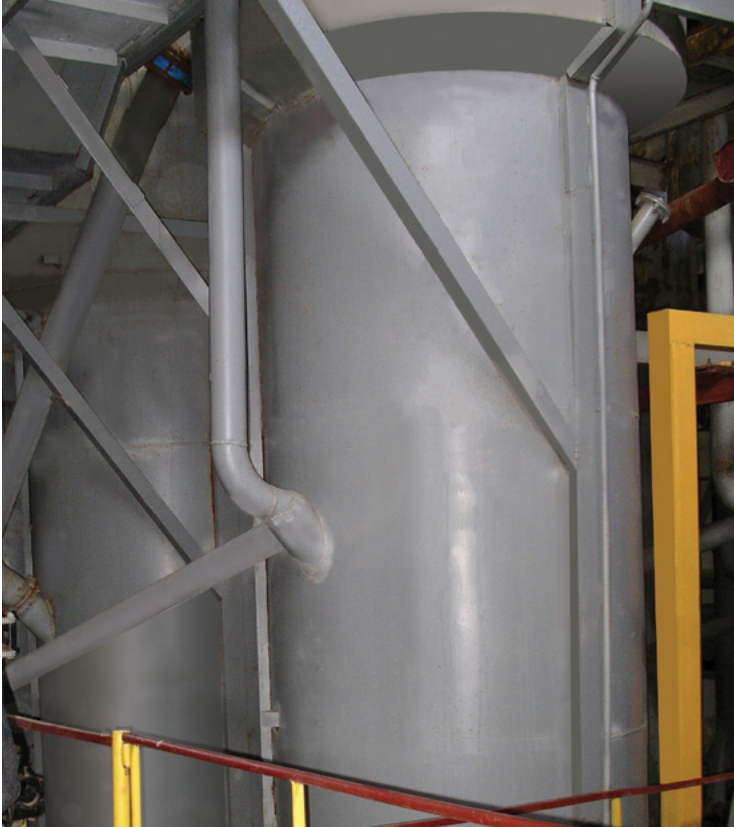
Fluidized bed ion exchange columns
